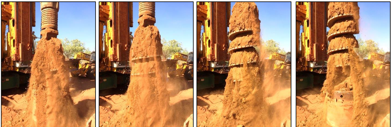
Figure 11: Sequence (from L-R) of Shallow Mineralisation Being Lifted from Bauer Hole THBA005, August 2015.
