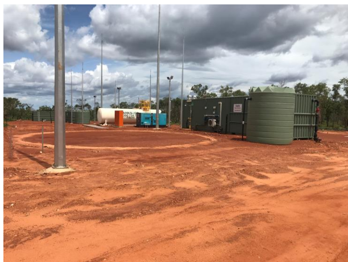
Waste water treatment plant at Thunderbird Village.
