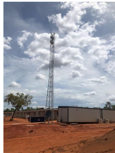
Communications infrastructure at Thunderbird Village.
